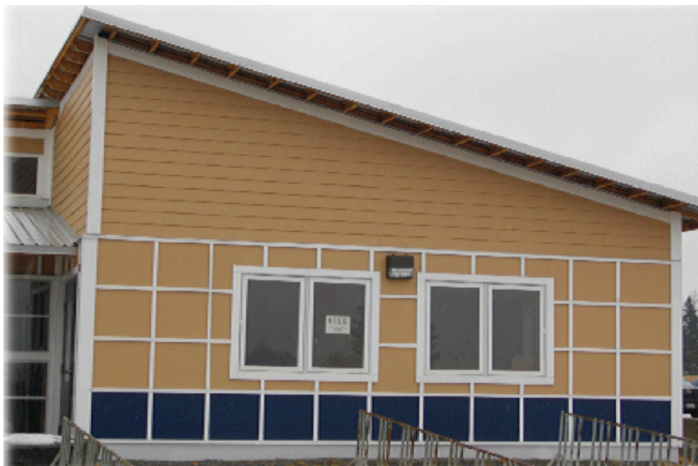
Figure 2: Elevation View EHI Demonstration, Lakehead University 2004-2006 Source: Chow K., Cotton C. and Deemter, M. (2010)
