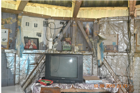
Fig. 9. Interior of Kaho's aid house showing no ceiling and soffit linings, author September 2013
