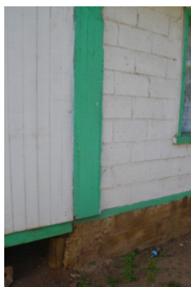
Fig. 4. Junction between Sioeli's cyclone house's timber stumps and concrete block addition's perimeter wall, author September 2013
